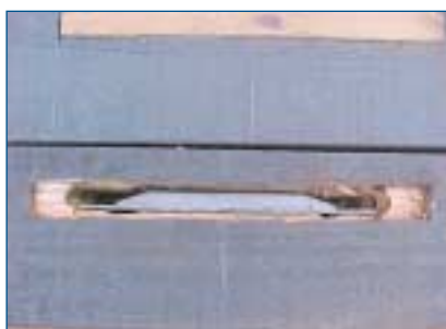
CVRD is using these 235 x 60 x 19 mm balises from Alstom, concealed within the sleepers, to provide train location data for its new train control system on the Carajás Railway, in conjunction with non-augmented GPS
