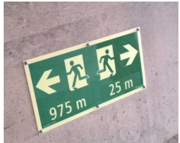
Signs will show passengers the distance to the nearest portal and the escape shaft. Photo BLS.
