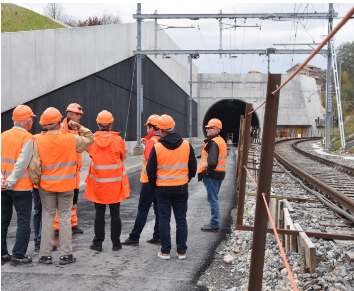
At the east portal, Markus Sägeser describes the challenges of the still-trackless Rosshäusern Tunnel. The existing line, which sees six trains per hour, is on the right.
