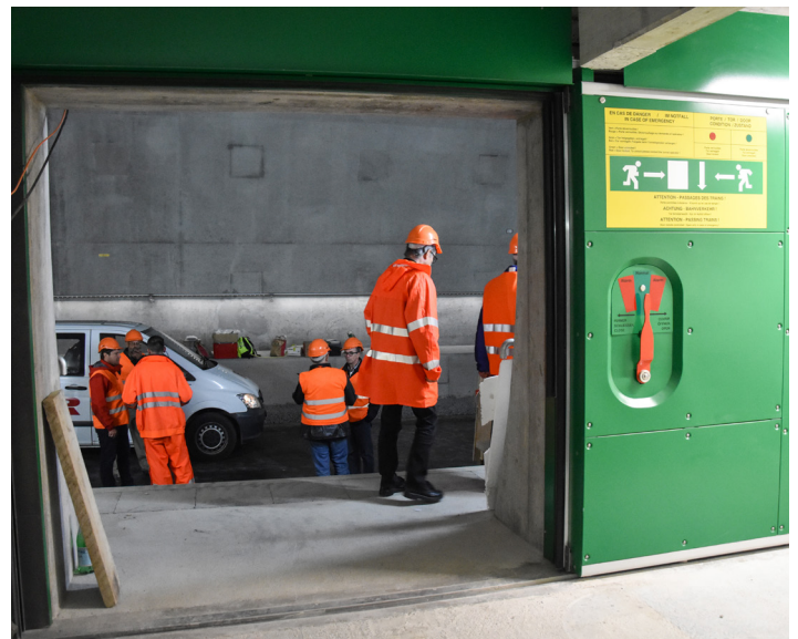
The tunnel has not received its tracks, but the access door to the 50 m high escape shaft at the tunnel's midpoint already bears labels in three languages. All photos George Raymond.
