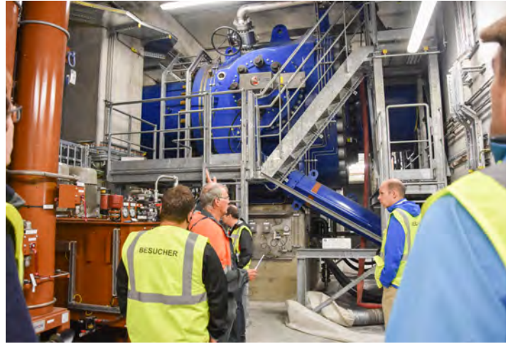
huge machines and complex control system; that huge physical forces (water volumes and speeds) are mastered; and that the dimensions and output of the whole plant are impressive.
