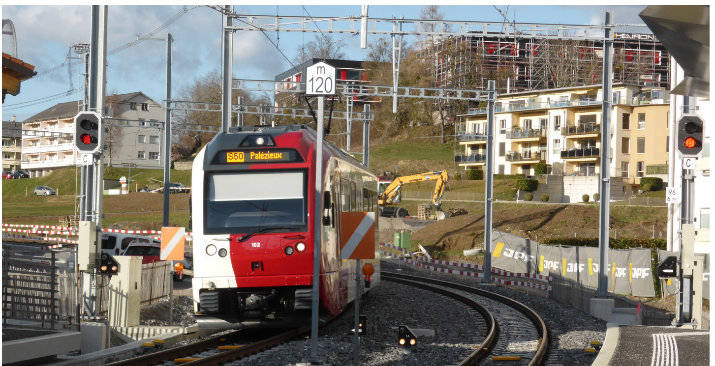
Châtel-St-Denis station on 6 March 2020. Some construction was still under way. All photos Daniel Pixley except as noted.
